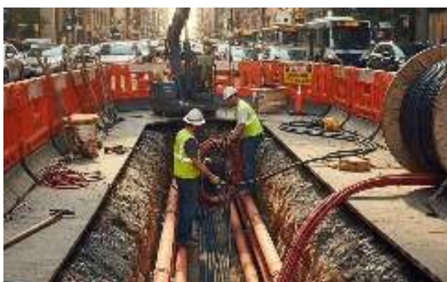
Underground Power Supply
